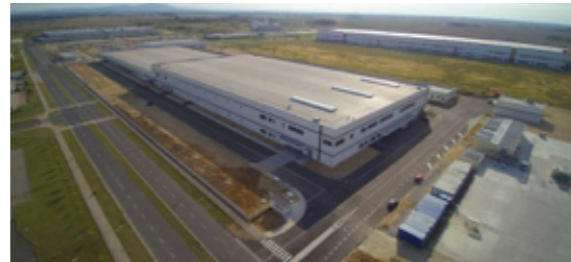
Project Name : LGESWA Dry Room Construction Client : LGEnergy Solution (Wroslaw, Poland) PJT Period : 2019~Processing
