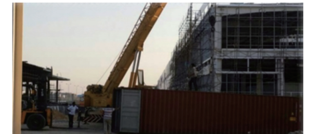
Project Name : LG ELECTRONIC CLEAN ROOM Construction Client : GS E&C (Egypt) PJT Period : 2013 ~ 2014
